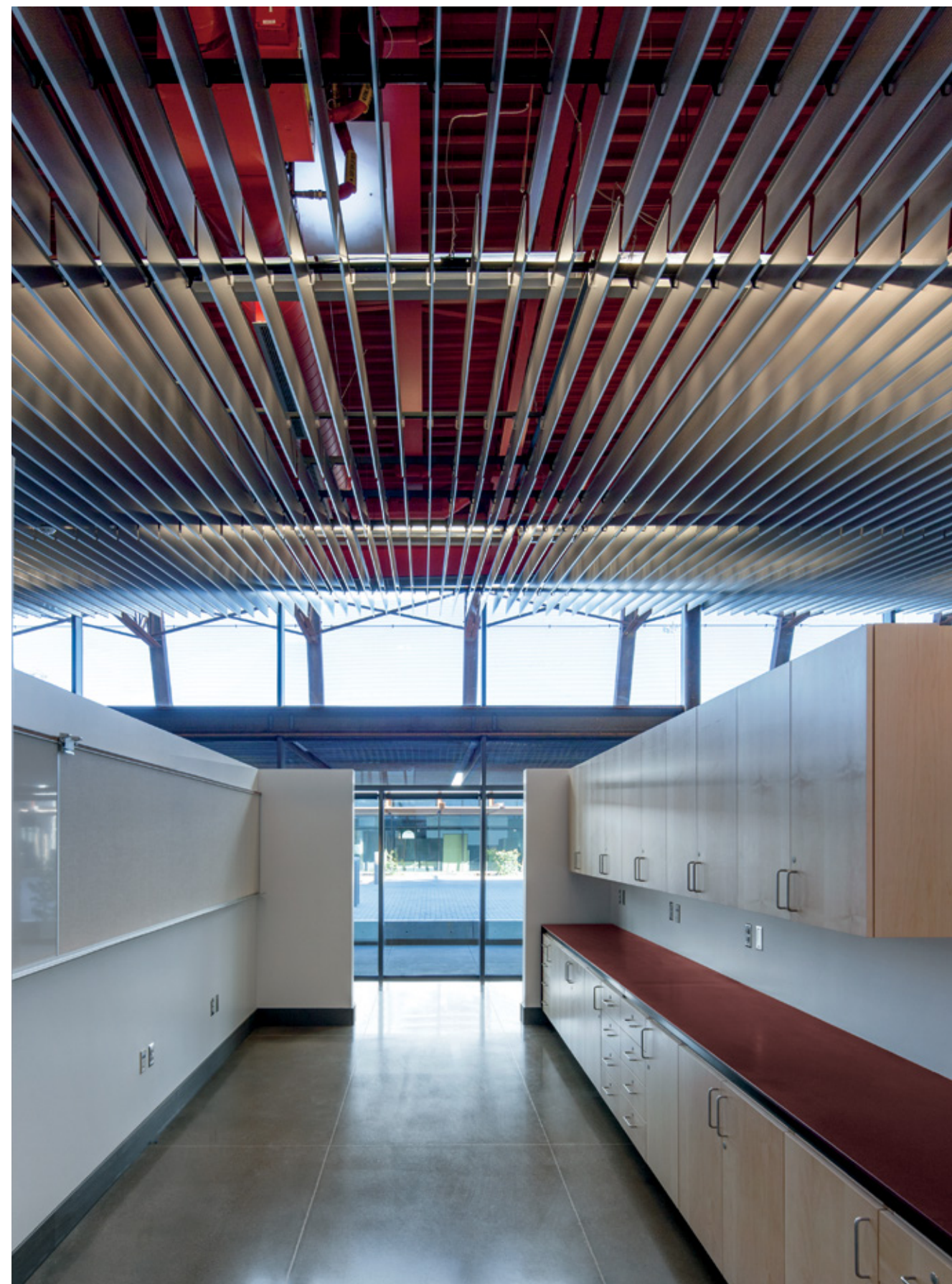
Project: Mariposa Land Port of Entry, Phoenix, AZ; V-Baffle Fins Photo credit: Bill Timmerman
