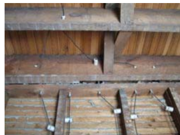
Fig. 2 - Knob and tube wiring in ceiling
