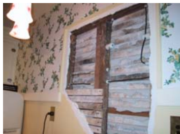
Fig. 3 - Knob and tube wiring in walls
