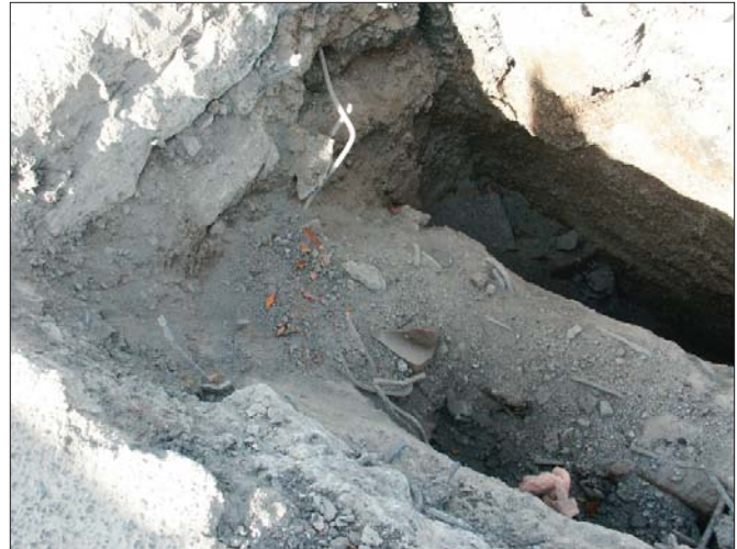
A portion of the project entailed the installation of a new 12-in. waterline — 500 ft in length — under an old freeway right of way.
