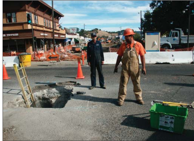
The North Marin Water District is proactively replacing its dated waterlines before a future pipe failure creates the necessity to dig up new city streets and sidewalks that are being planned.
