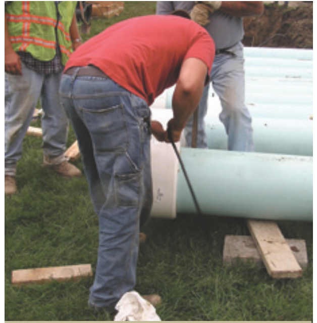
A worker ties a nylon spline to a section of Certa-Lok restrained joint pipe, preparing it for installation.
