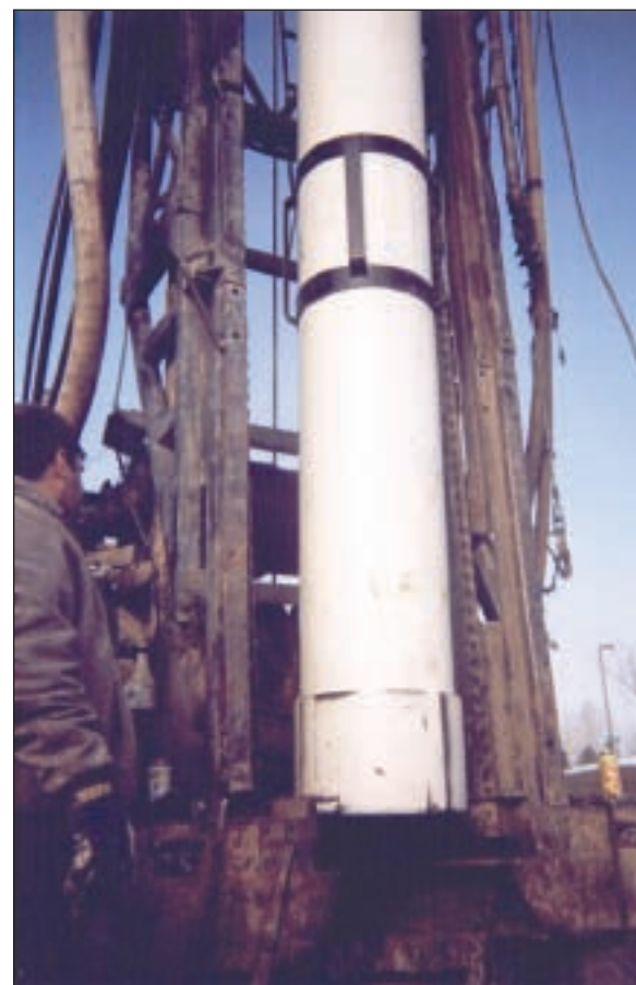
A 17-inch PVC casing is ready for installation in a new supply well in Meridian, Idaho.
