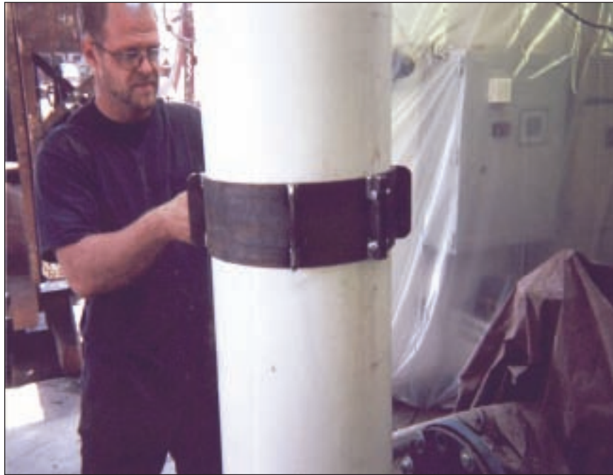
Dave McLeran, owner of McLeran Well Drilling LLC in Fruitland, Idaho, prepares a PVC casing to be installed as the new lining in a corroded, old steel well in Meridian, Idaho.
