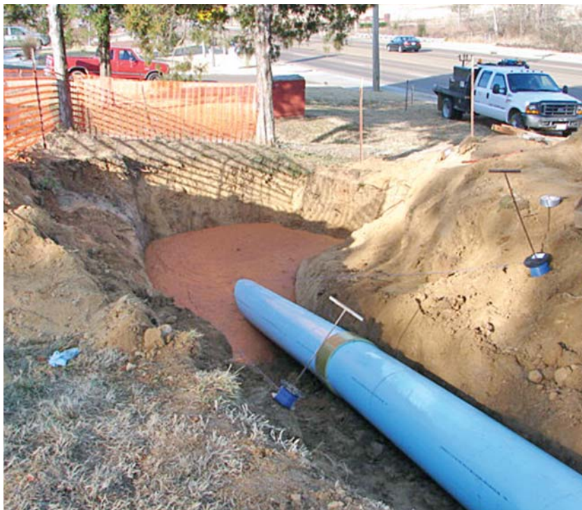
Top: Memphis Boring and Tunneling's and Revell Construction's drilling crew prepare to ream a bore for a new water transmission line in Oakland, TN.
