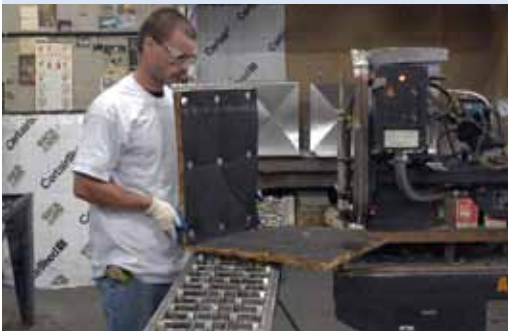
Fiber glass duct liner is pinned to sheet metal during the fabrication of a sheet metal duct.
