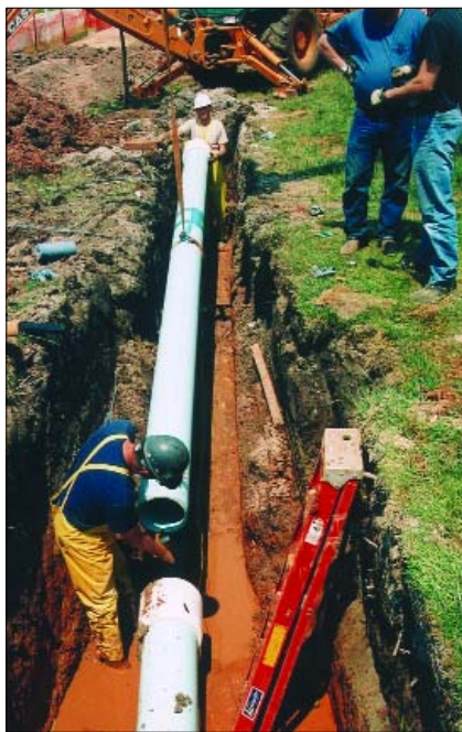
Workers connect lengths of CertainTeed C900/RJ pipe as part of Missouri State University's new chilled water system.
