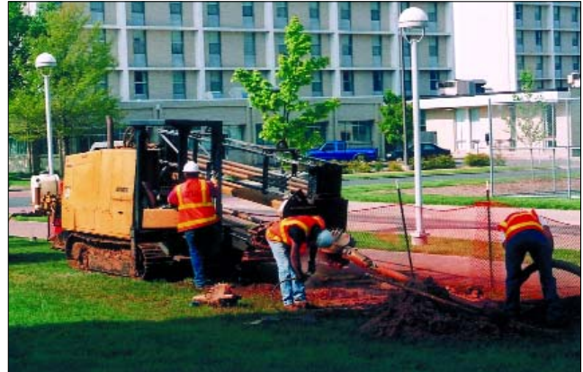
Workers prepare to pull pipe for Missouri State University's new chilled water system.
