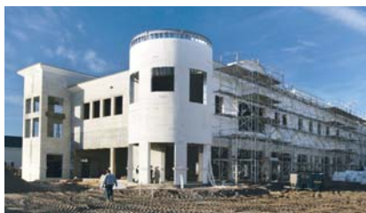
Sikon Construction scaffolding sits ready for EIFS installers who, according to Project Superintendent Jason Rice, "prefer CertainTeed's GlasRoc ® Sheathing. EIFS foam, applied with specially formulated adhesive, bonds to CertainTeed's GlasRoc ® Sheathing better than yellow board, and it's harder to pull off. With CertainTeed's GlasRoc ® Sheathing, the bond is stronger."
