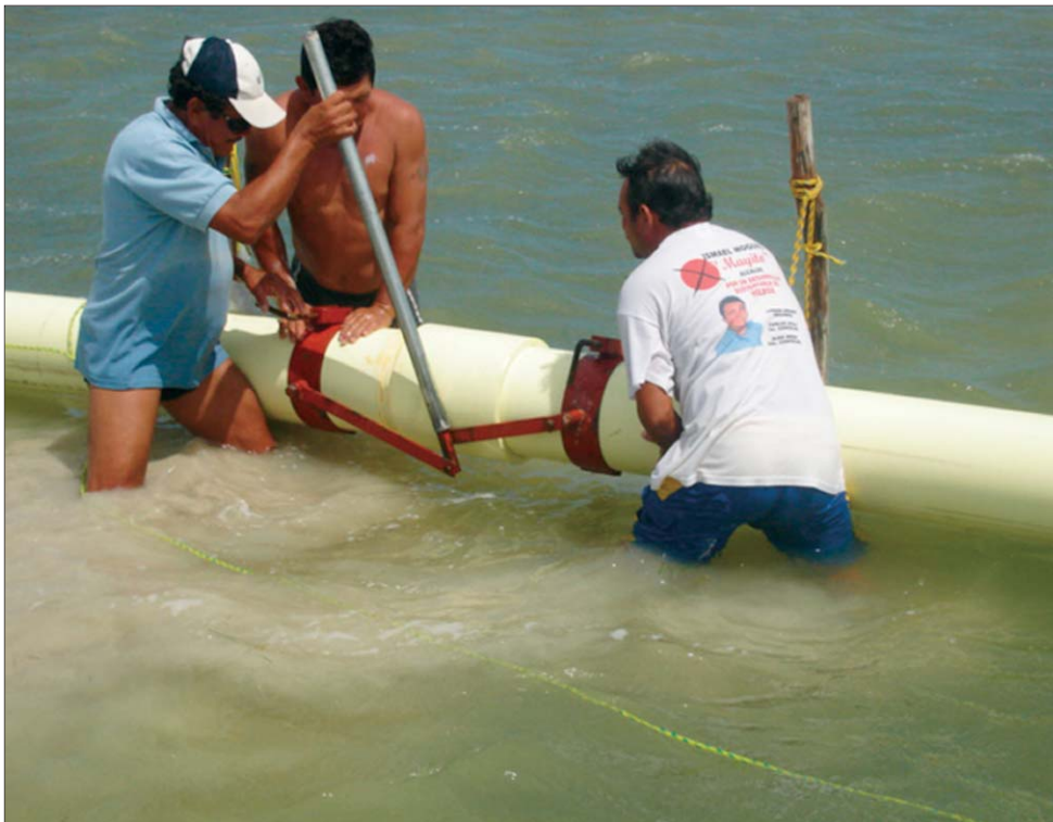
Because of the difficult and unusual environment, the engineer designed and used a special lever system tool to help assemble the pipe.
