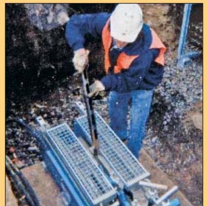
Quicklock bursting rods are linked together, not screwed together, like traditional drill stems or other static systems. This system speeds the installation process as well as the breakdown procedure. The rods can be quickly removed one at a time at the exit pit as bursting is in progress.
