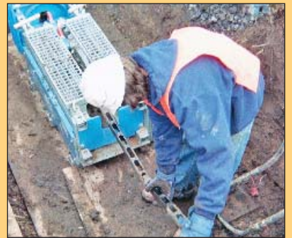
The Grundoburst's specially designed bladed rollers makes bursting difficult host pipe like ductile iron and steel possible. In this case, CNC crews replaced 1,300 lf of 8-inch steel irrigation main with the static system.
