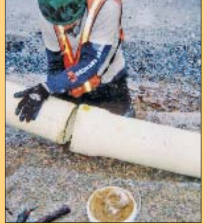
The CNC crews utilized the Grundoburst static pipebursting system that allowed them to use a restrained joint PVC product pipe. The Certa-Lok Yelomine PVC pipe assembled easily as the bursting operation proceeds, without the need for special fusion equipment.
